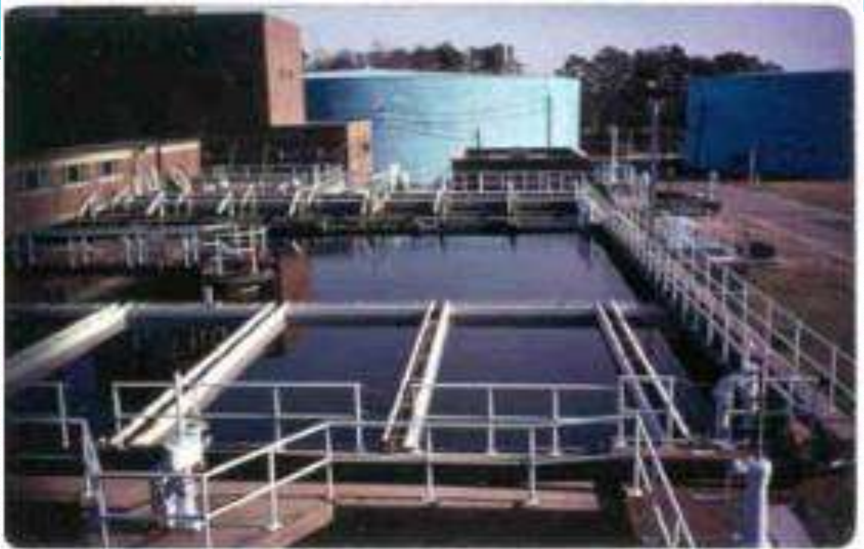
A rectangular settling tank
